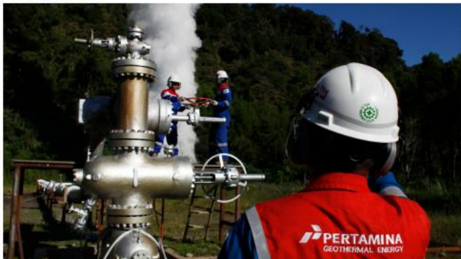
PT Pertamina Geothermal Energi workers rotate a valve at Karaha geothermal well in Tasikmalaya, Indonesia. The Southeast Asian nation's geothermal potential is second in the world only to the U.S. © Reuters
