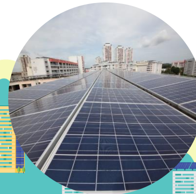
Solar Panels on Rooftops
