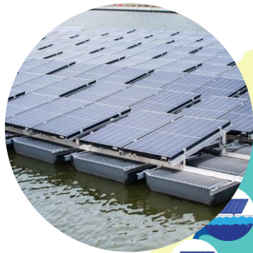
Floating Solar Modules
